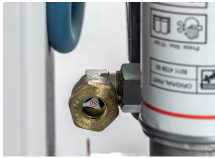
Oil level check
