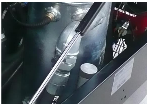
Figure 10.1-1 Checking the oil level in the compressor
