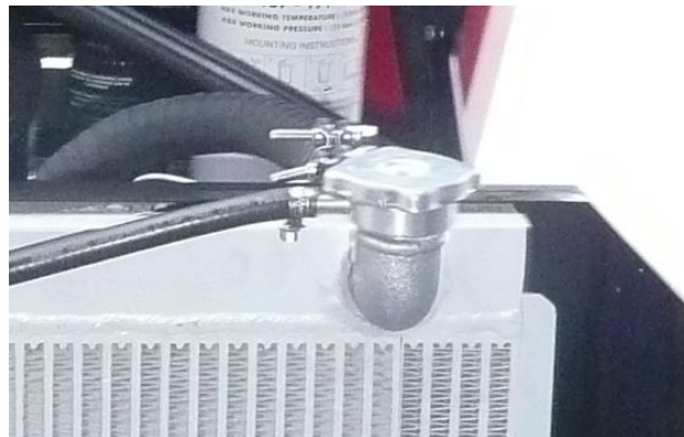
Figure 13.4-3 Checking the coolant radiator
