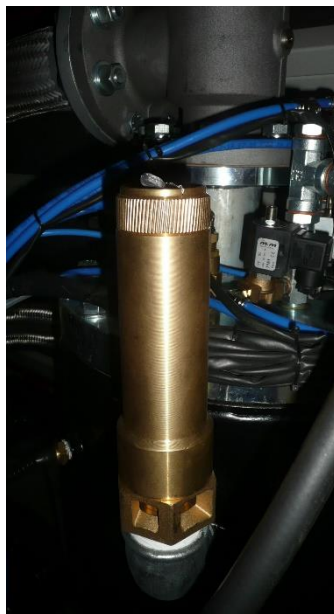
Figure 12.2-1 Control of the safety valve
