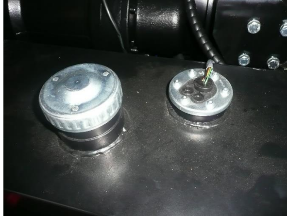
Figure 10.1-2 Gas oil tank for Diesel engine
