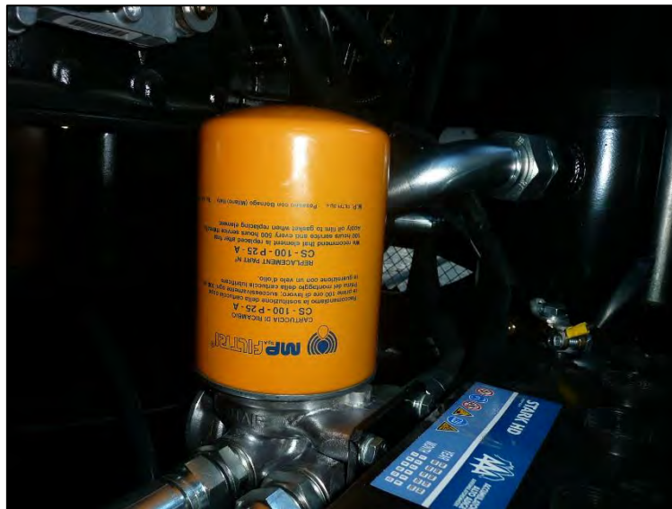
Figure 13.4-5 Compressor oil filter
