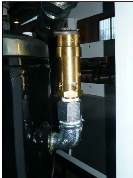
Figure 12.1-1 Control of the safety valve
