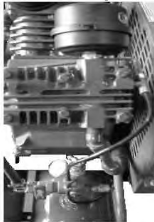
Unloader line to spray
